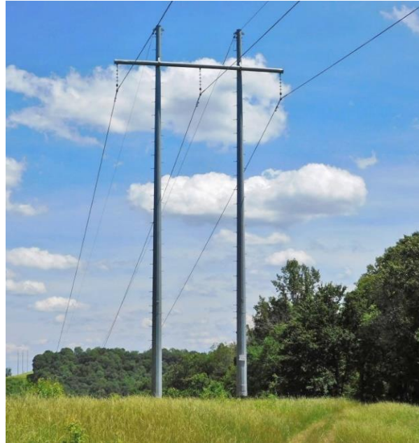
Figure 2. Typical Transmission Line Structure (Steel H-Frame) approximately 80 feet tall (average).
