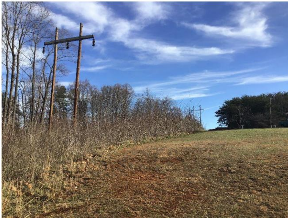
Photo 4. City of Danville's Pinnacles – Hydro 69-kV Transmission Line
